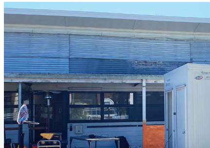
Cladding (approx. 74 sqm), guttering and worn downpipes need replacing at the front of our Foundation Centre
