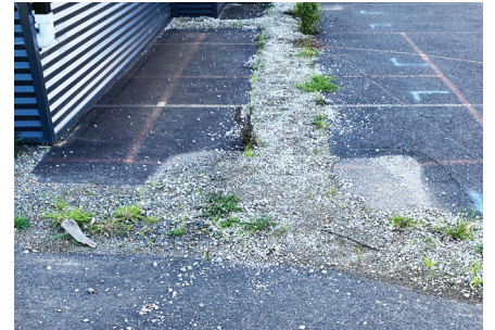
Broken asphalt at our Discovery Centre needs to be repaired
