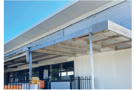
Our Foundation Centre verandah requires sanding and repainting
