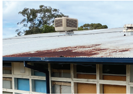
Roofing (approx. 102 sqm) needs to be replaced in a rusted section at our Foundation Centre
